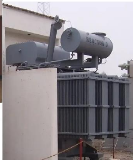
REACTOR MARCONA 5 MVar, 10 kV
